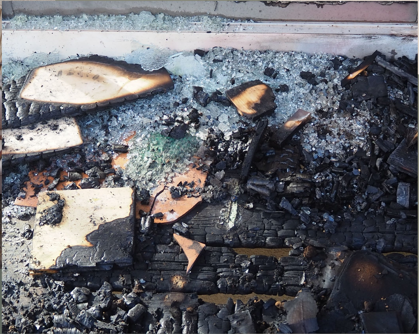
FIRE INVESTIGATION – Topki Drive
